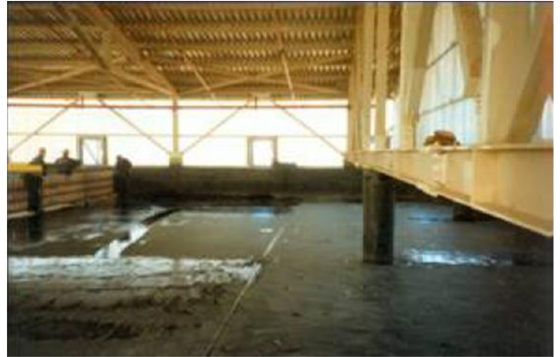
SX tanks used to effect a separation of a warm mixture of sulphuric acid and an aggressive organic liquid (similar to kerosene) into its two components
