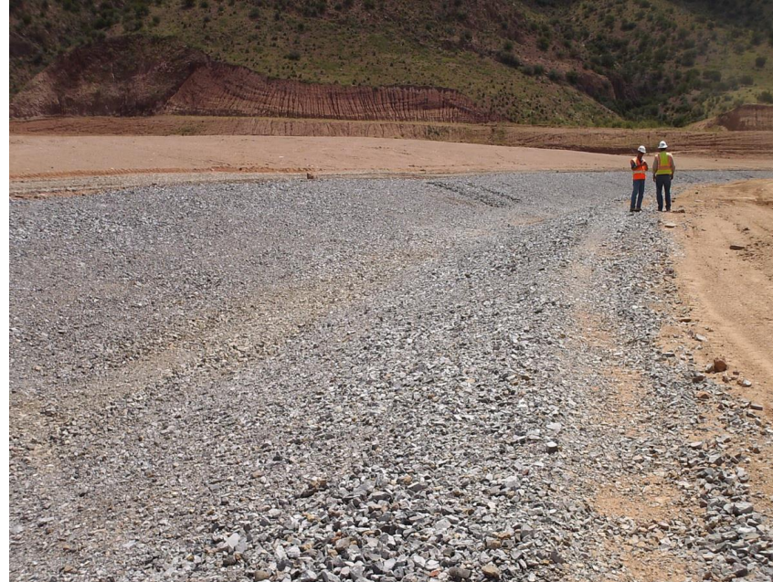
Geocell storm water channel
