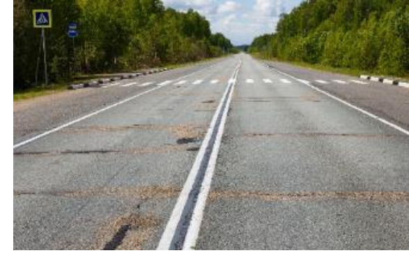
Reflective Cracking from expansion joints
