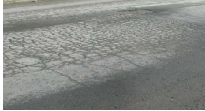
Alligator Cracking due to structural failure
