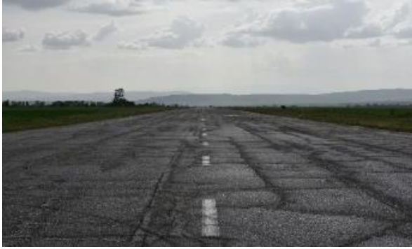
Reflective cracking from concrete bays
