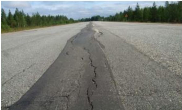
Temperature Cycles Reflective Cracking
