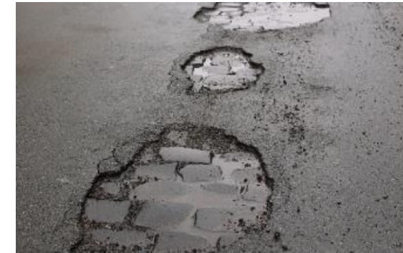
Surfacing failure caused by underlying setts
