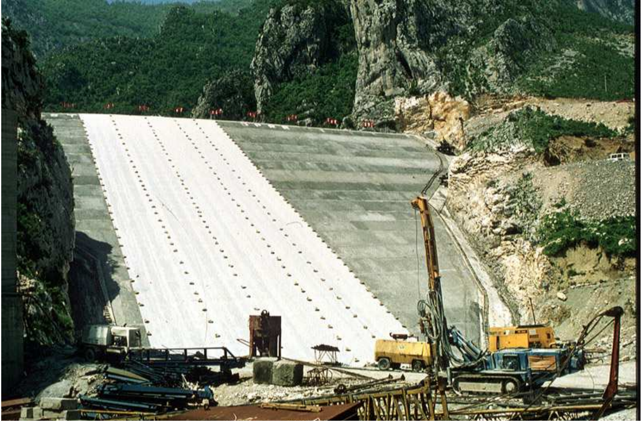
An extra layer of PP nonwoven geotextile (800 g/m 2 ) was placed over the composite geomembrane before the casting of unreinforced concrete slabs
